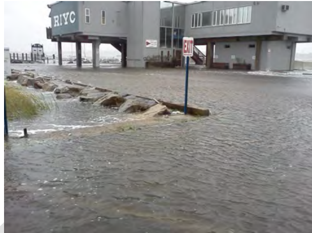
Hurricane Irene caused road damage in 2011. Photo credit: Cranston Patch
